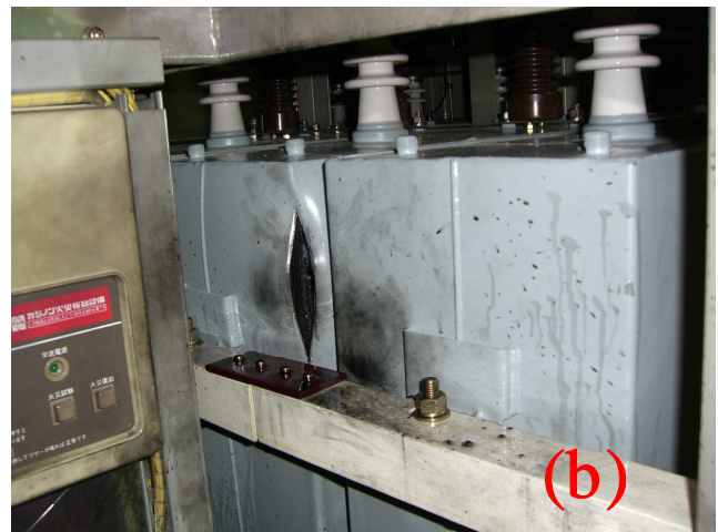
Fig. 4. (a) HPLT_D and oil leakage (b) Burst Capacitor
